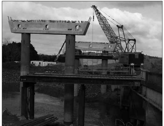
"Bridge to Nowhere" - precast bridge can be bolted together with virtually no 'on site' concrete.
